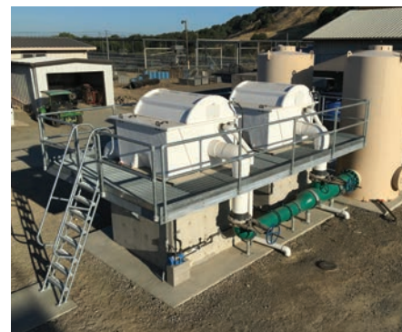
Facilities such as the Nimbus Hatchery in California utilize recirculation technology to reduce water demand and improve biosecurity.
