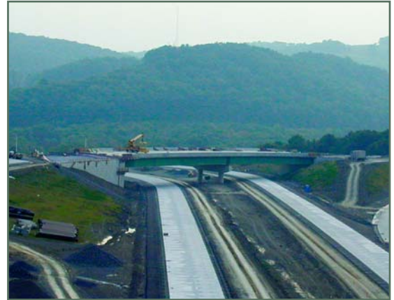
With its unequal length curved spans, Bridge 207 was a good candidate to observe global twisting behavior.
