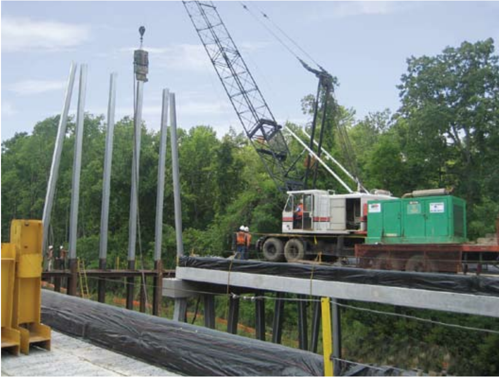
Top-down construction in action — construction over the wetlands area progressed at an average of one span per week.
