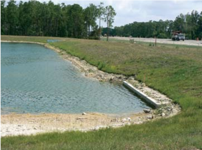
Triple 48-inch pipes (foreground) provide inflow to the pond. A control structure can be seen in the far corner.
