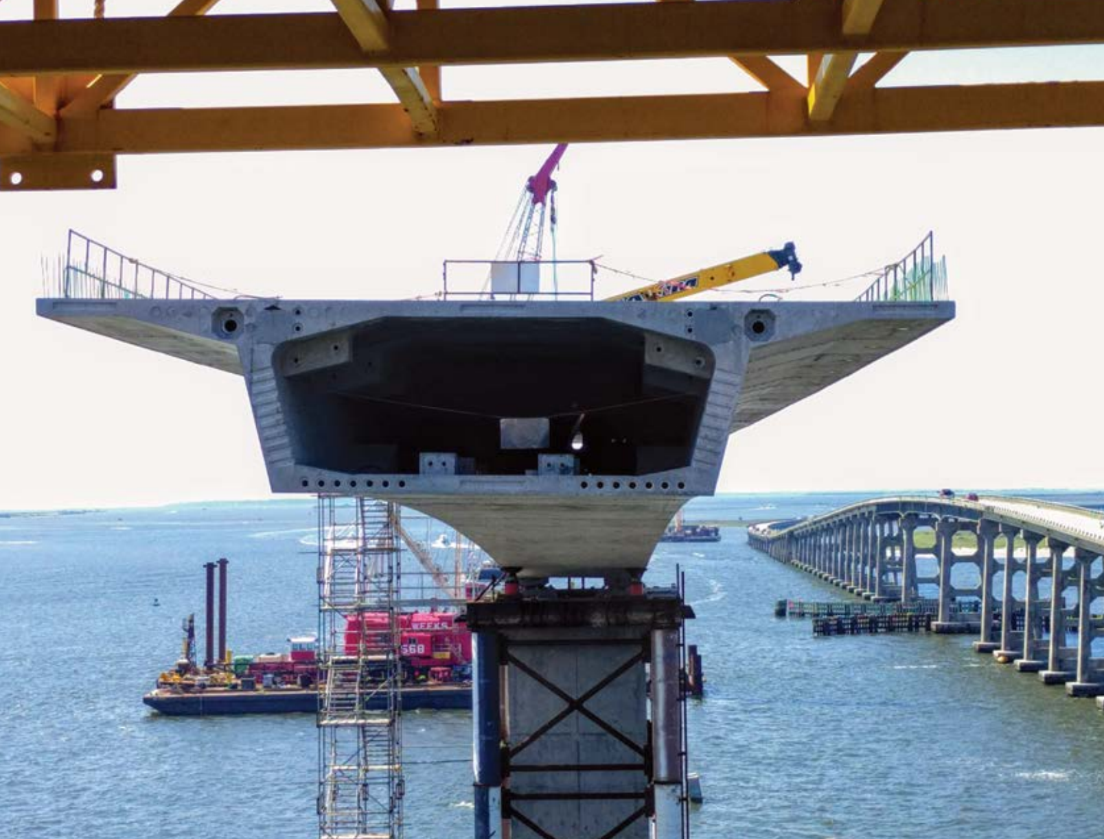
The new Bonner Bridge incorporates a balanced cantilever design featuring a wide variety of precast concrete products.
