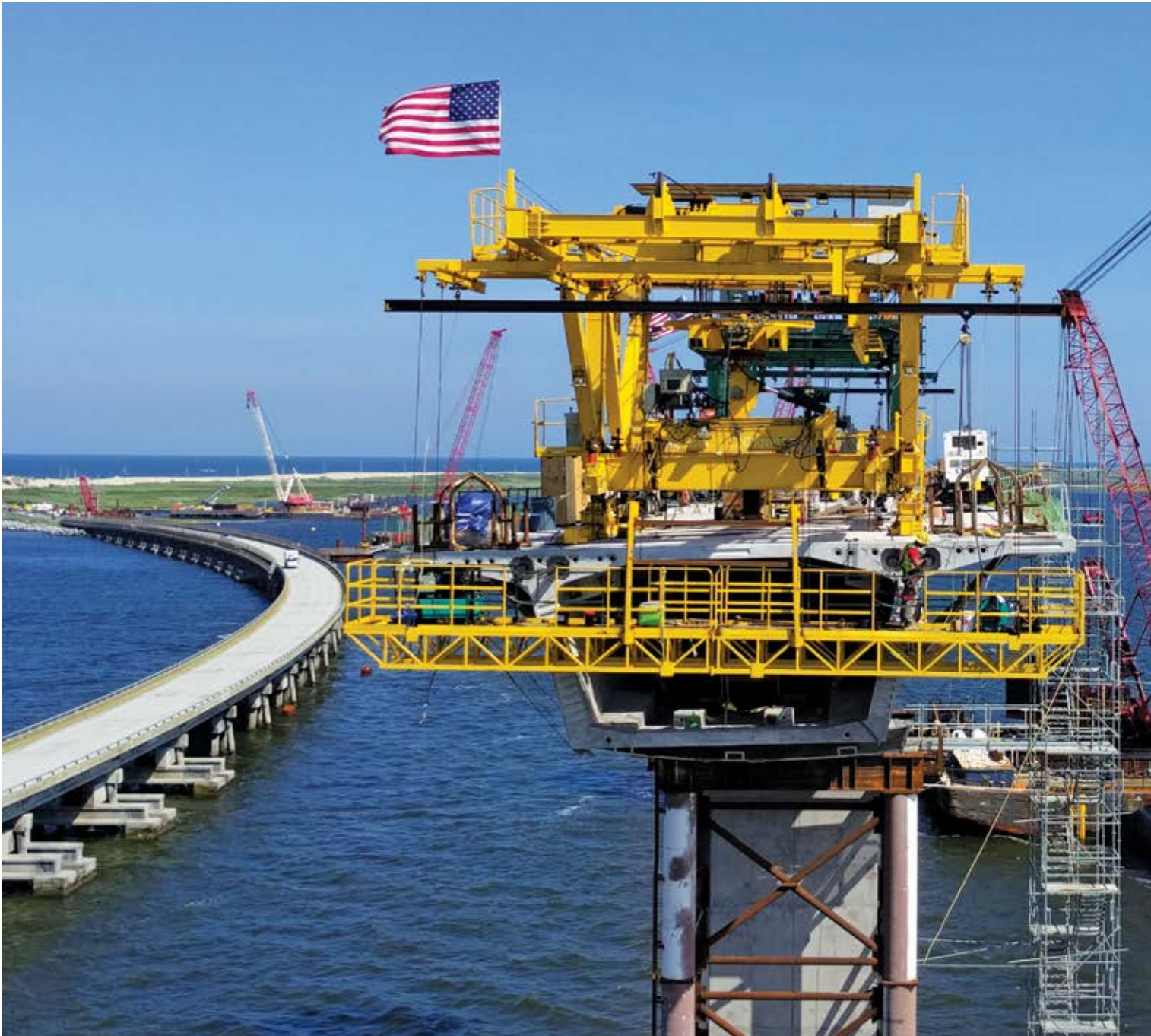
Thanks to the use of precast, the new Bonner Bridge will boast a 100-year service life.
