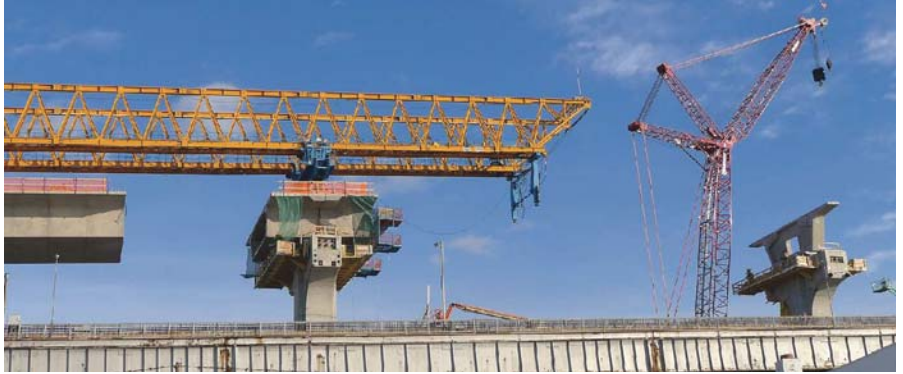
Gantry erection of cantilever at expansion pier and split-pier segment erection by crane.
