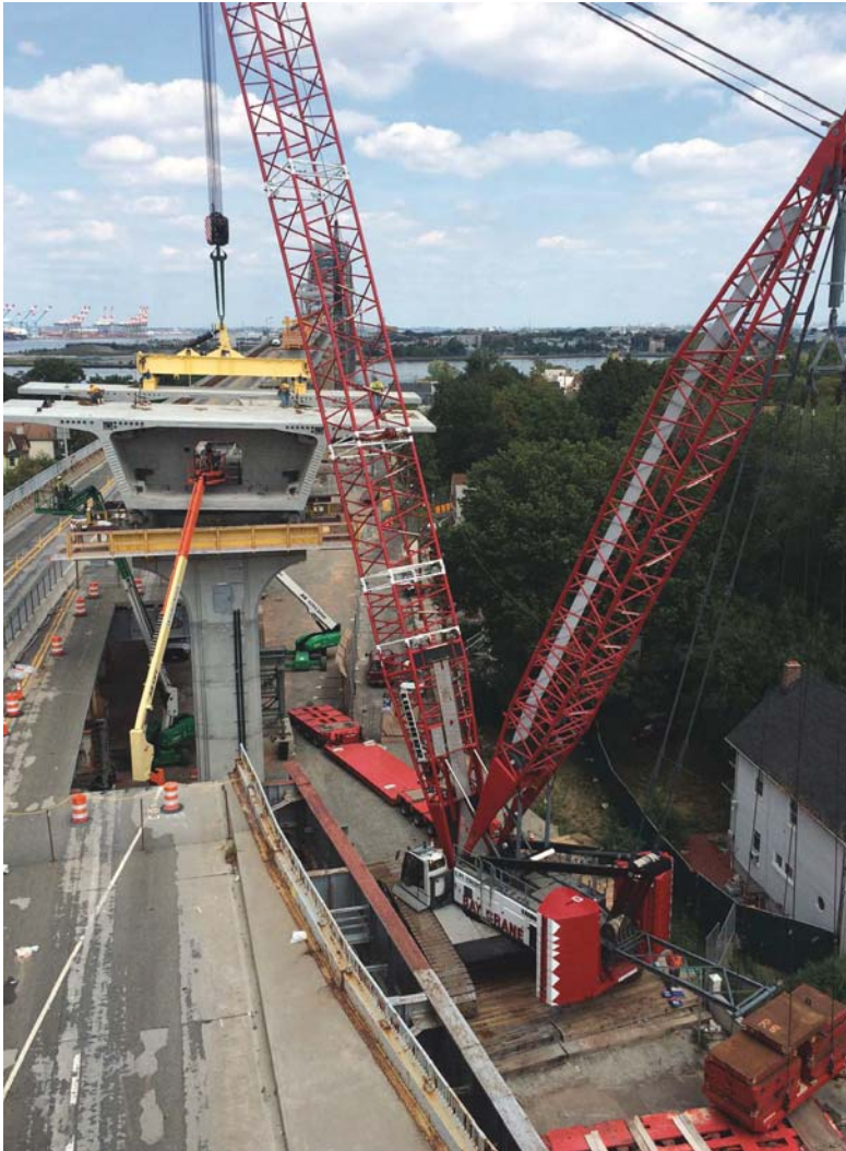
Tight constraints for erection of single-cell box-girder pier table segment. The 42-ft difference in the elevations of the old and new approaches is evident. All Photos and Figures: HDR.
