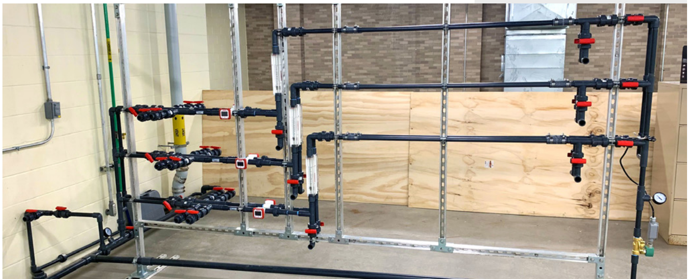
Figure 3. City of Cedar Rapids Pipe Rig Unit Showing Three Test Rigs
